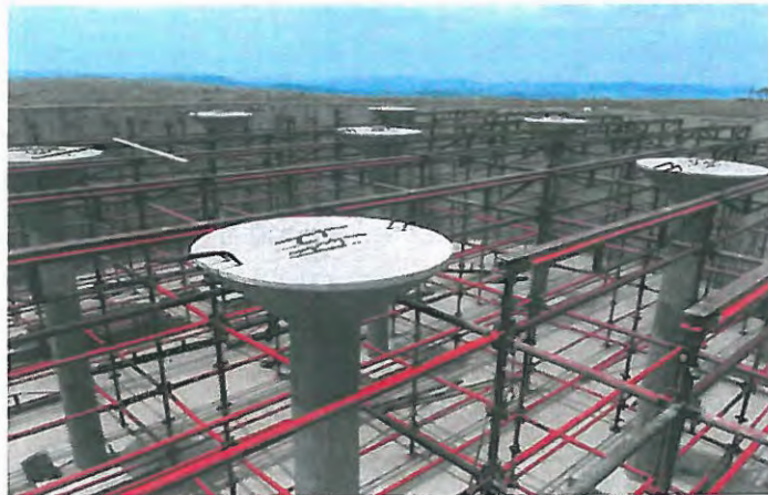
CONSTRUCTION OF A 5 ML RESERVOIR AT ROOF LEVEL FOR SIMDLANGENTSHA EAST RWSS
